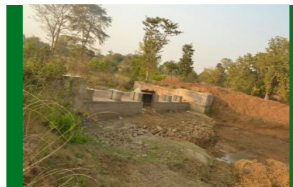
Sluice Valve For the Check Dam
