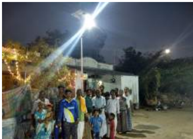
Photo: Solar street light installed in village common place
